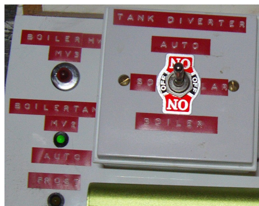
ABOVE – Diverter Switch: UP = AUTO CENTRE= SOLAR TANK OUTPUT DOWN = BOILER TANK OUTPUT
